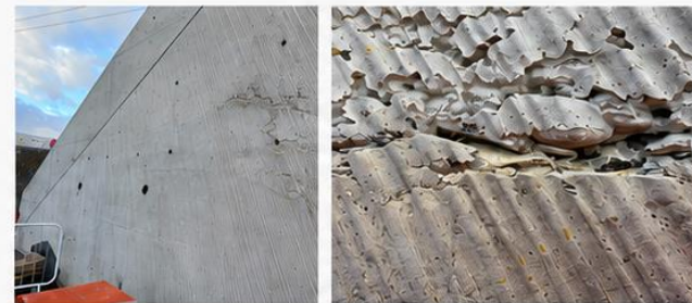
Severe defects – honeycombing and voids
