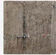
Cracking mapped and measured.
